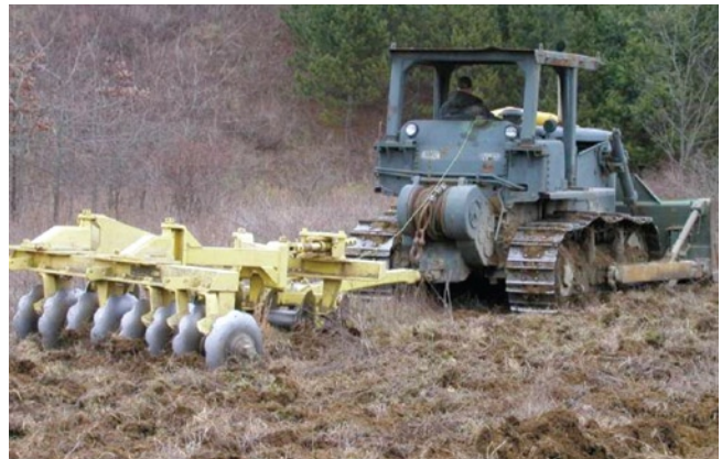
Figure 8. A large disk being used to break up surface soil and herbaceous vegetation root mass prior to soil ripping. This operation is not always necessary, but it can increase the efficiency of the deep tillage operation on sites where dense vegetation is present.
