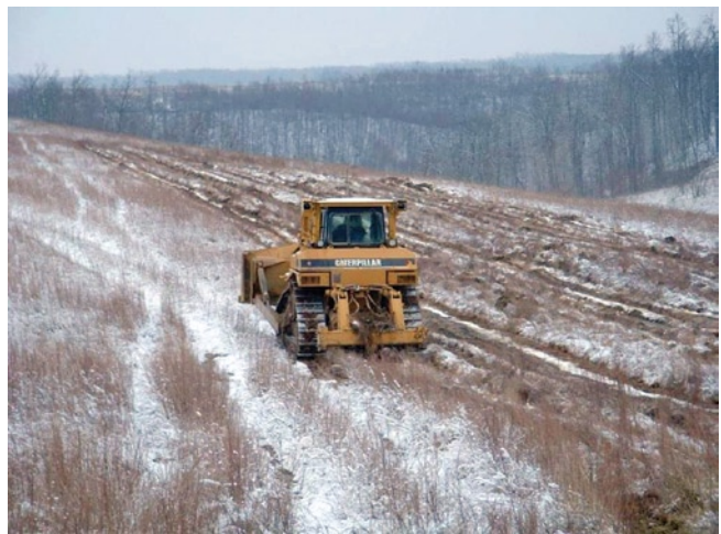
Figure 5. A standard single-shank ripper preparing a mine site for reforestation. The soil-ripping “tooth” being pulled by the dozer is intended to loosen soil material to a depth of 3 feet or more. The best results are achieved if this operation is performed in late summer and fall when the soil is dry.
